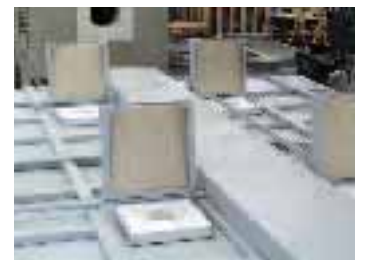
Automatically controlled vapour vent flaps
