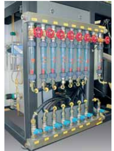
Cooling water supply
