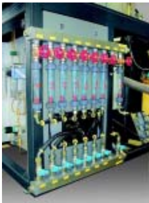
Cooling water supply
