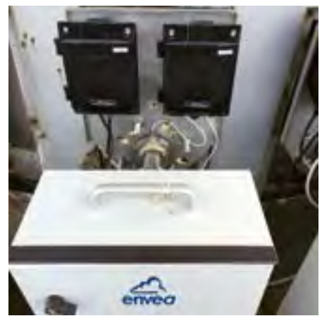
STACK OR DUCT ONLINE MONITORING
