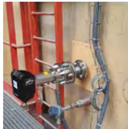
CROSS DUCT, INLINE COMBUSTION MONITORING
